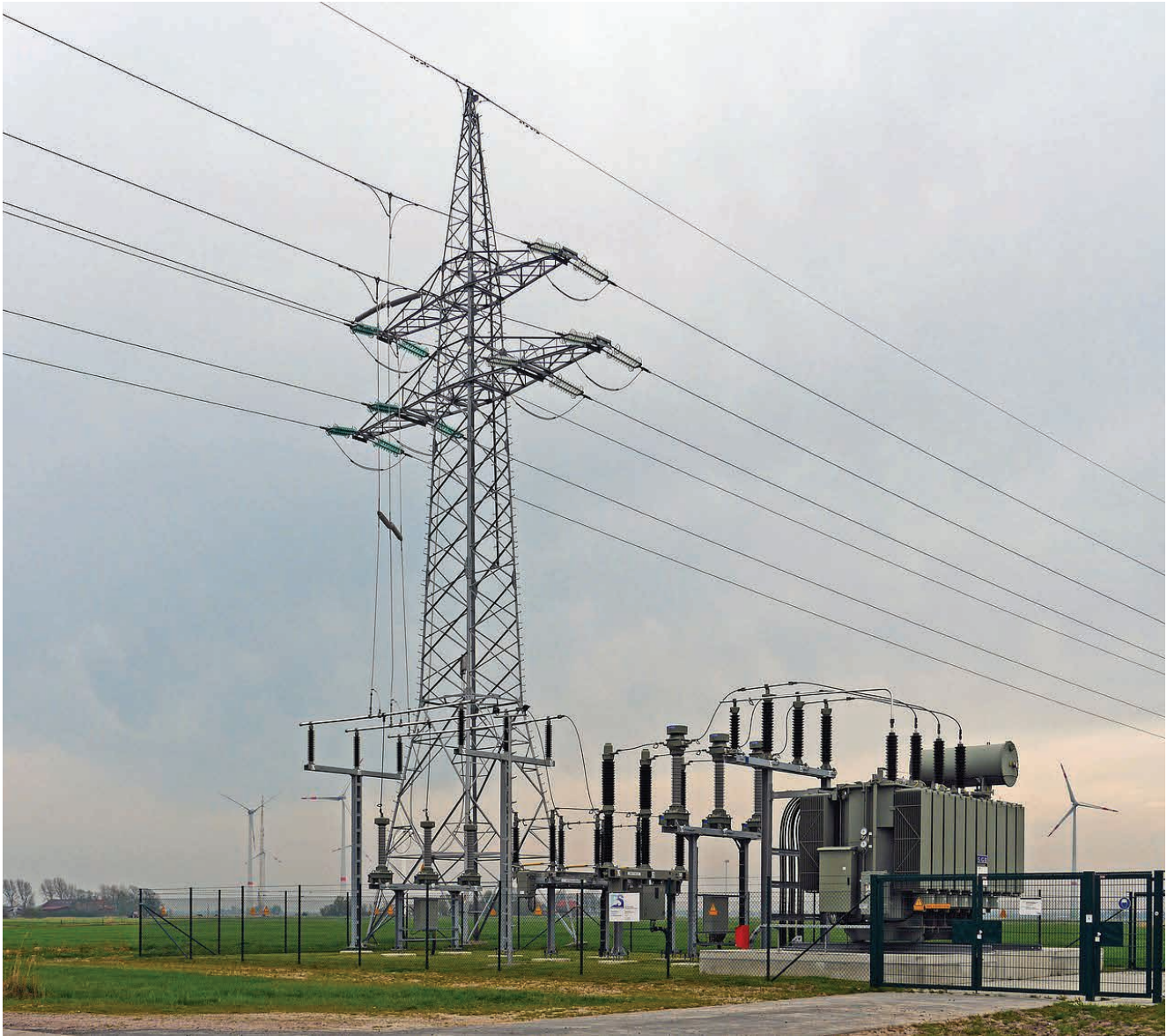
En example of a 72kV vacuum circuit breaker installation, copnnecting a renewable energy plant with a transmission network.
